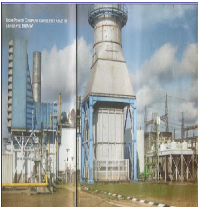
Fig.1. The Ibom Power Plant shows the transformers, transmission and distribution networks of the plant courtesy of Ibom Power plant project website.
